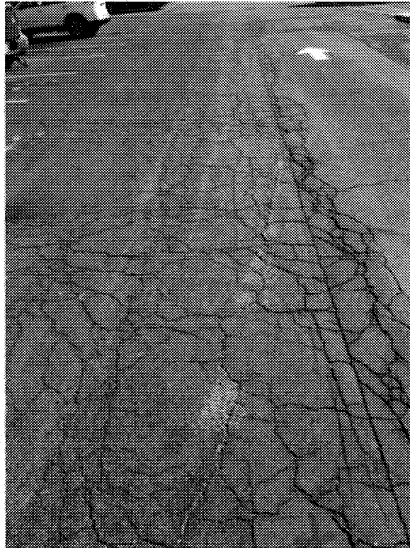
Pavement Distress Photograph 1 - Grid 3
